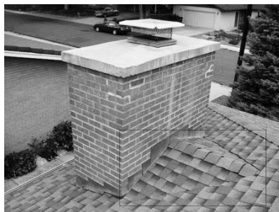
Clay Liner Cover
